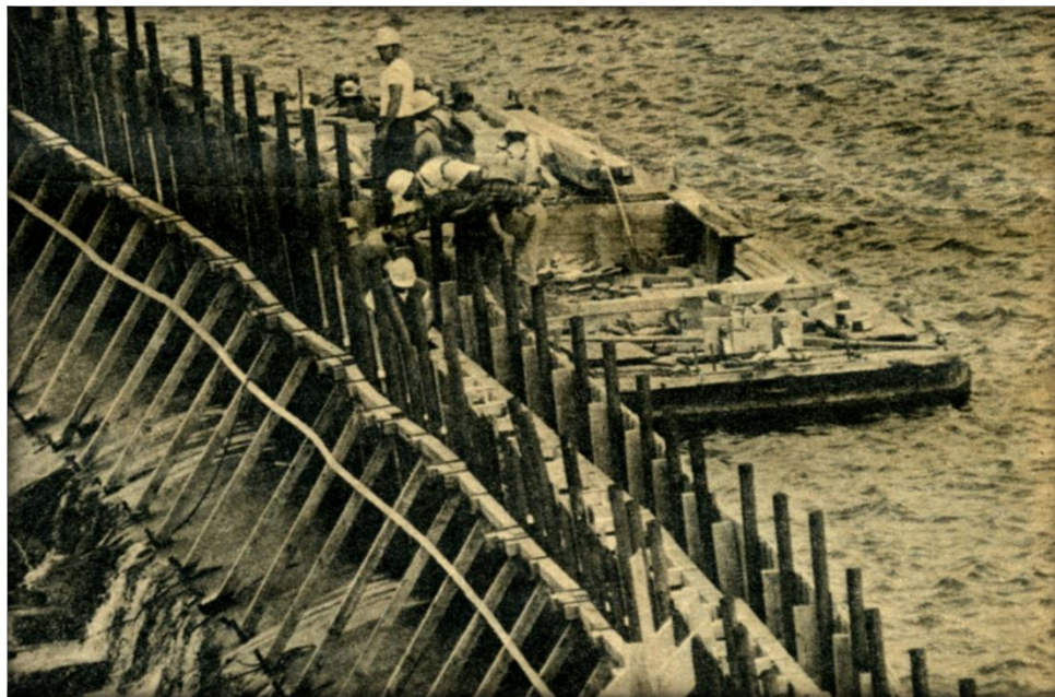
Hydro-maintenance crew build flashboard* structure to facilitate work at Montague Dam. It will be topped by four plate steel hydraulic Bascule gates*, each 120 feet long by more than 13 feet high, believed to be the largest in the world.
