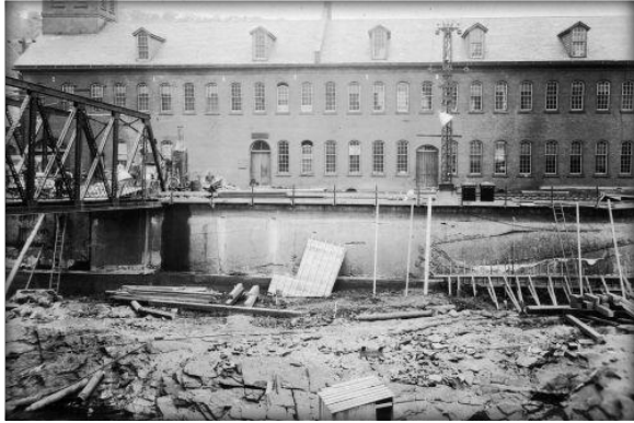
Canal wall at Russell Cutlery. Repairs are being made to the break in the wall. e.g. archive
